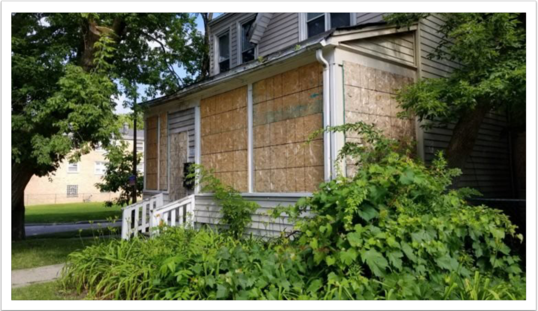
Image 1. Home in Evanston in need of repair
